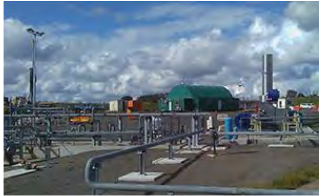
Figure 9. General view of the Huntly UCG pilot site
