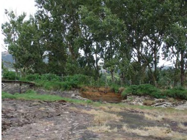
Photograph 4: Pond 1 Scarp on the inside Embankment
