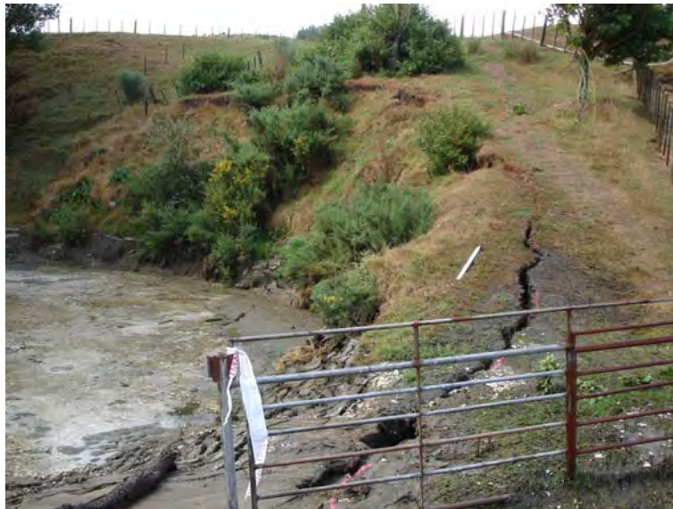
Photograph 3: Fissure Formation near the Sinkhole
