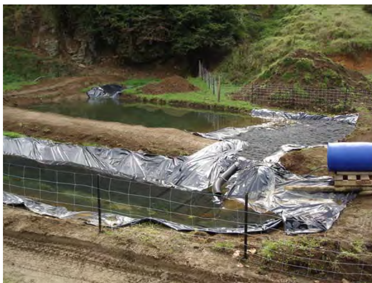
Photograph 5: Temporary Spring Flow Treatment System
