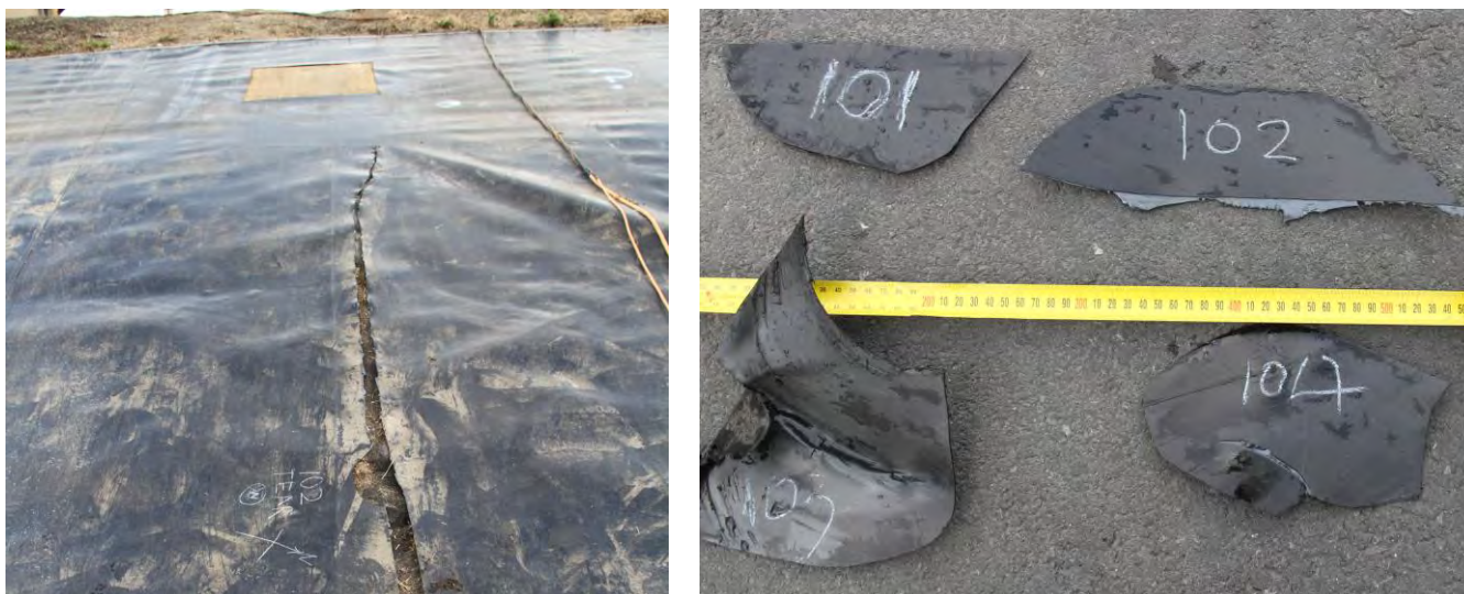
Photographs 1 & 2: Liner showing tear line, detailed damage of various areas and testing area
