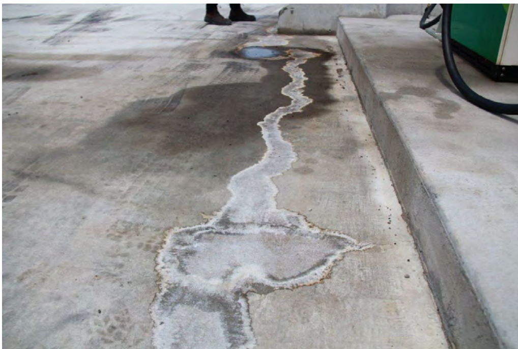
Photograph 1. Dried DEF on a forecourt.
